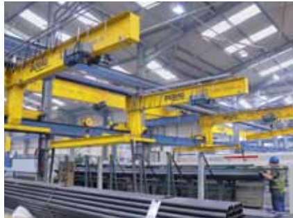
Wall-travelling cranes fitted with long-material spreaders serving production machinery
