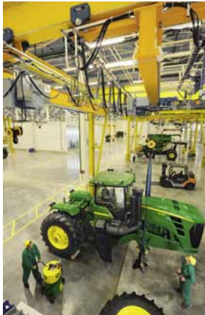
Station served by two 7.5 and 10 t suspension cranes
