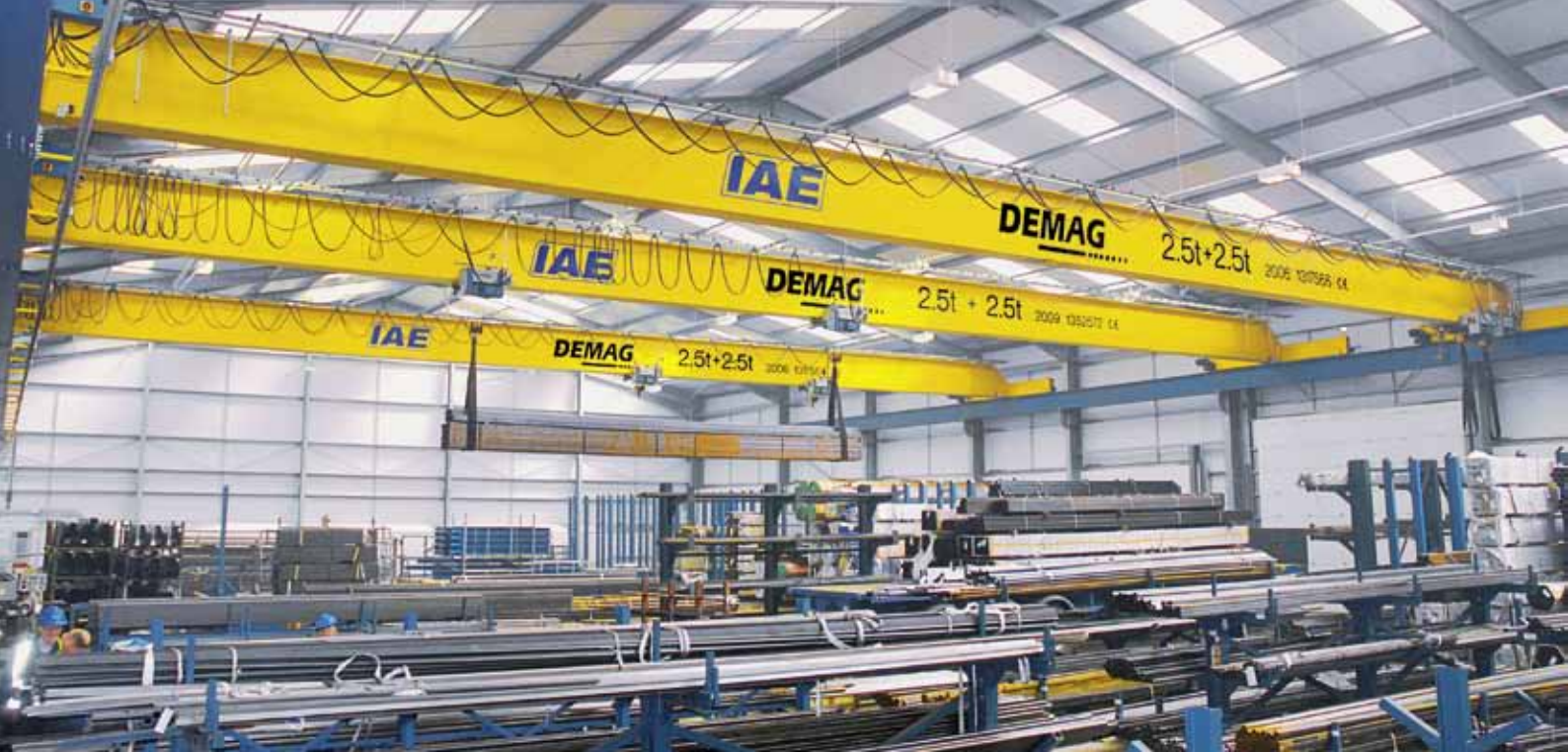
Three EKE overhead travelling cranes, each fitted with two 3.2 t wire rope hoists, operating on one runway in the storage facility
