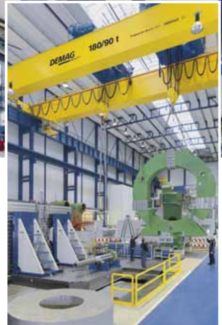
Process crane above the gantry
