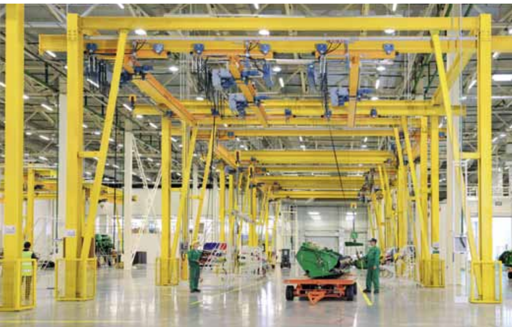
Assembly cells featuring steel superstructures with up to three suspension cranes
