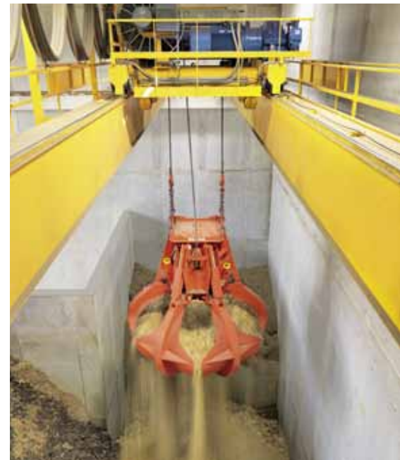
Filling the silo with solid fuel
